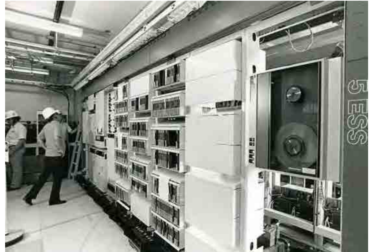
No. 5 ESS, Seneca, IL (1982) Photo courtesy AT&T Archives and History Center
