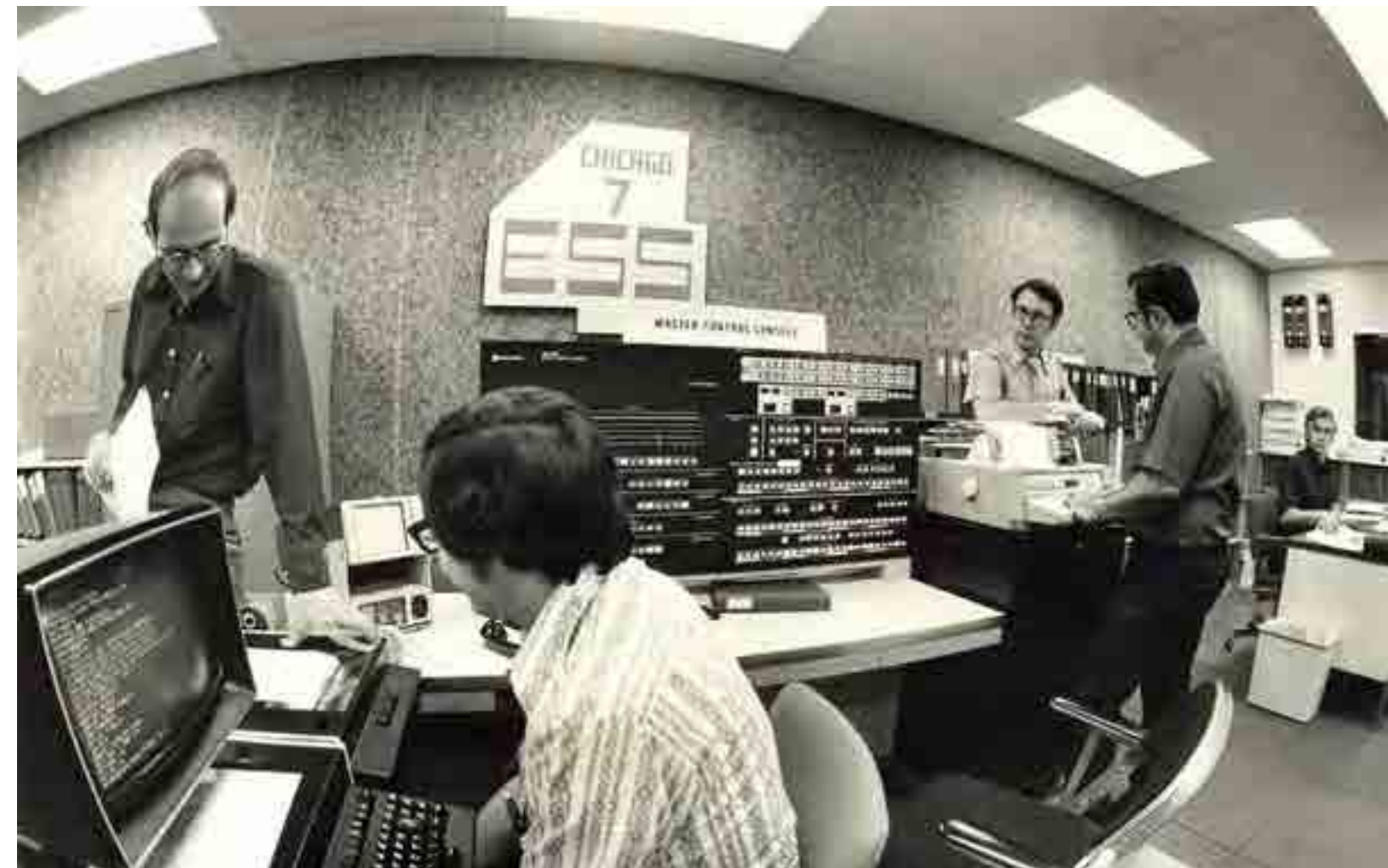
No. 4 ESS Installation, Chicago, IL (1975 - 1976) Photo courtesy AT&T Archives and History Center
